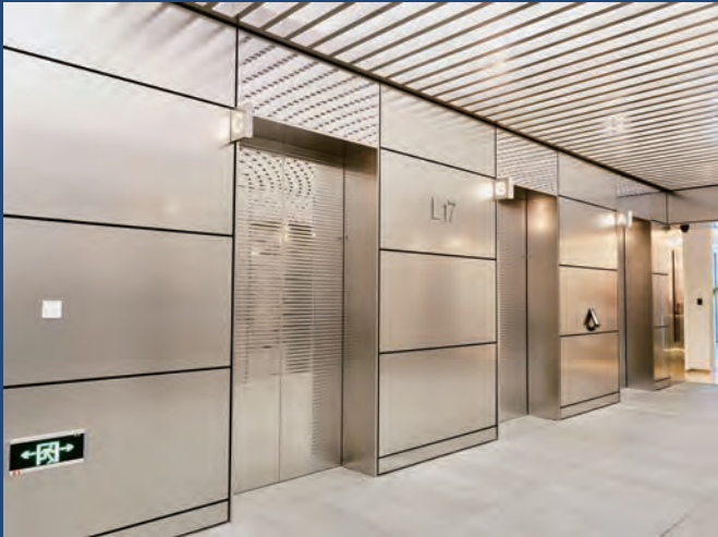
Elevators, Escalators and passenger conveyors
